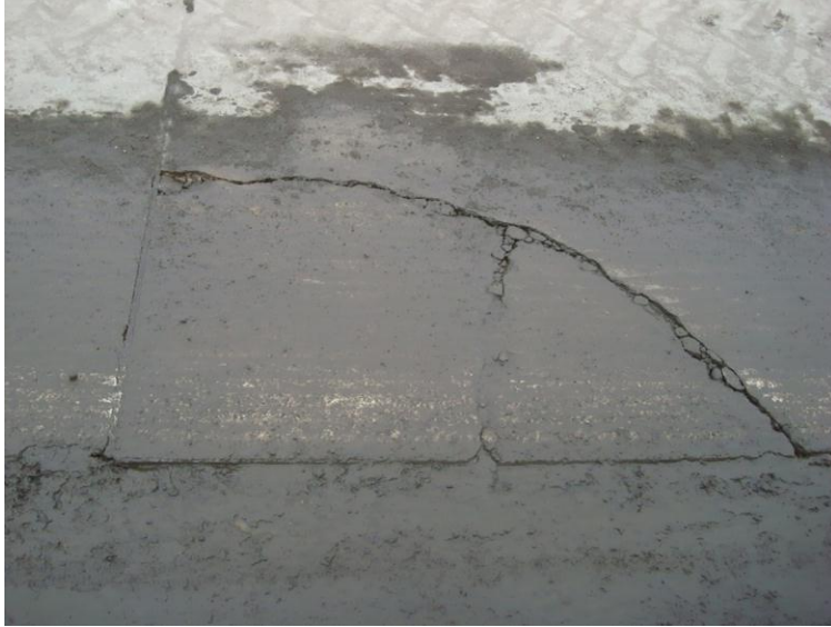
Figure 4-27. Aggravated Corner Break from Fall 2009 Testing Cycle
