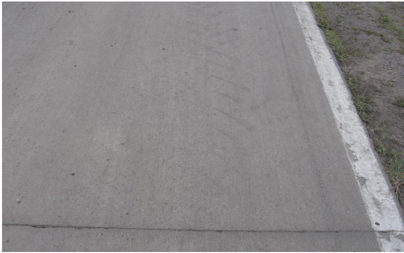
Figure 4-35. New Corner Break on Cell 32 during Fall 2010 Testing
